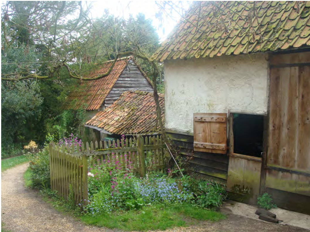
Picture 1.15 Former agricultural buildings within the curtilage of Aylward's, the roof of one building in particular is in need of repair
